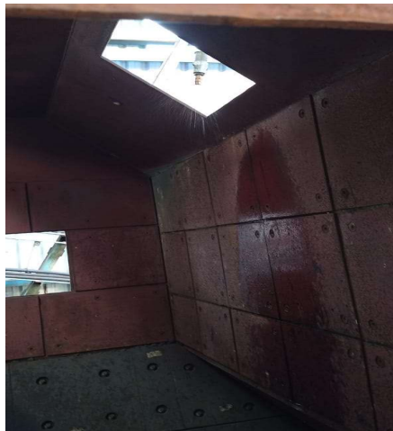
Sprinkler at transfer points
