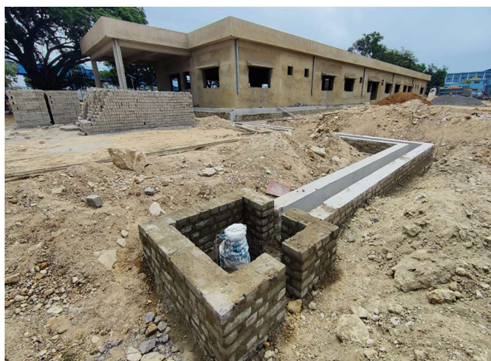
Ground water recharge system
